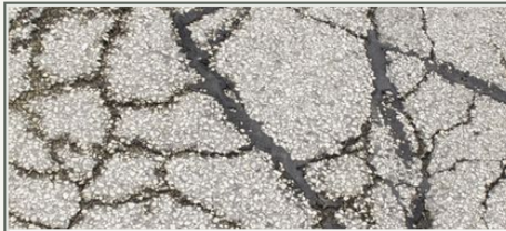
P-14 parking asphalt cracking
