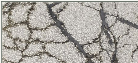
P-14 parking asphalt cracking
